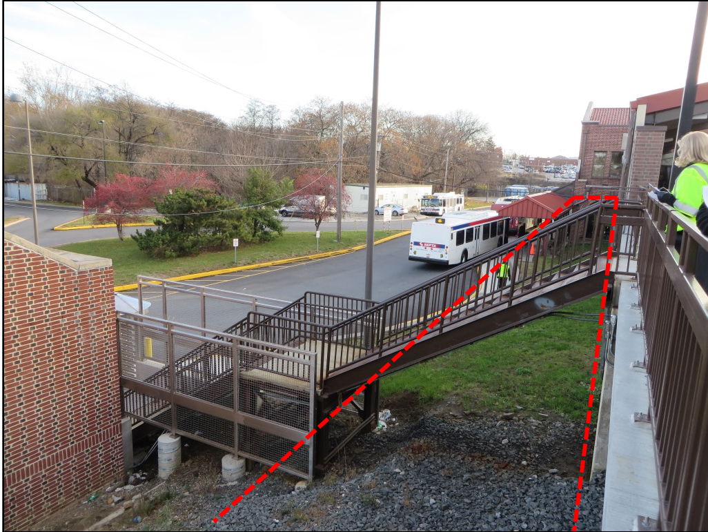
Photograph 17. View looking east along the exterior of the north platform at the 69 th Street Transportation Center, proposed location of new track and widened platform.
