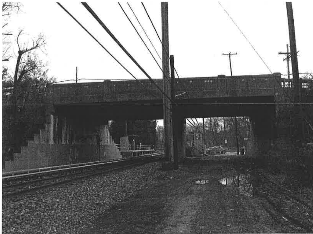
Photograph 3: Philadelphia and Western Railway, view facing south showing the Ardmore Avenue Bridge.
