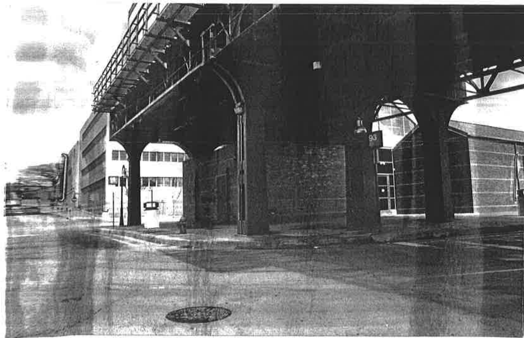
P hoto g r a ph 3: Detail, P&W trestle at its connection to the Norristown Transportation Center, facing northeast.
