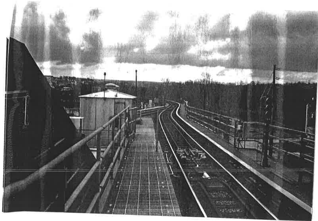
Photograph 8: P&W trestle, looking south from Norristown Transportation Center toward the viaduct that carries the line across the Schuylkill River into Bridgeport.
