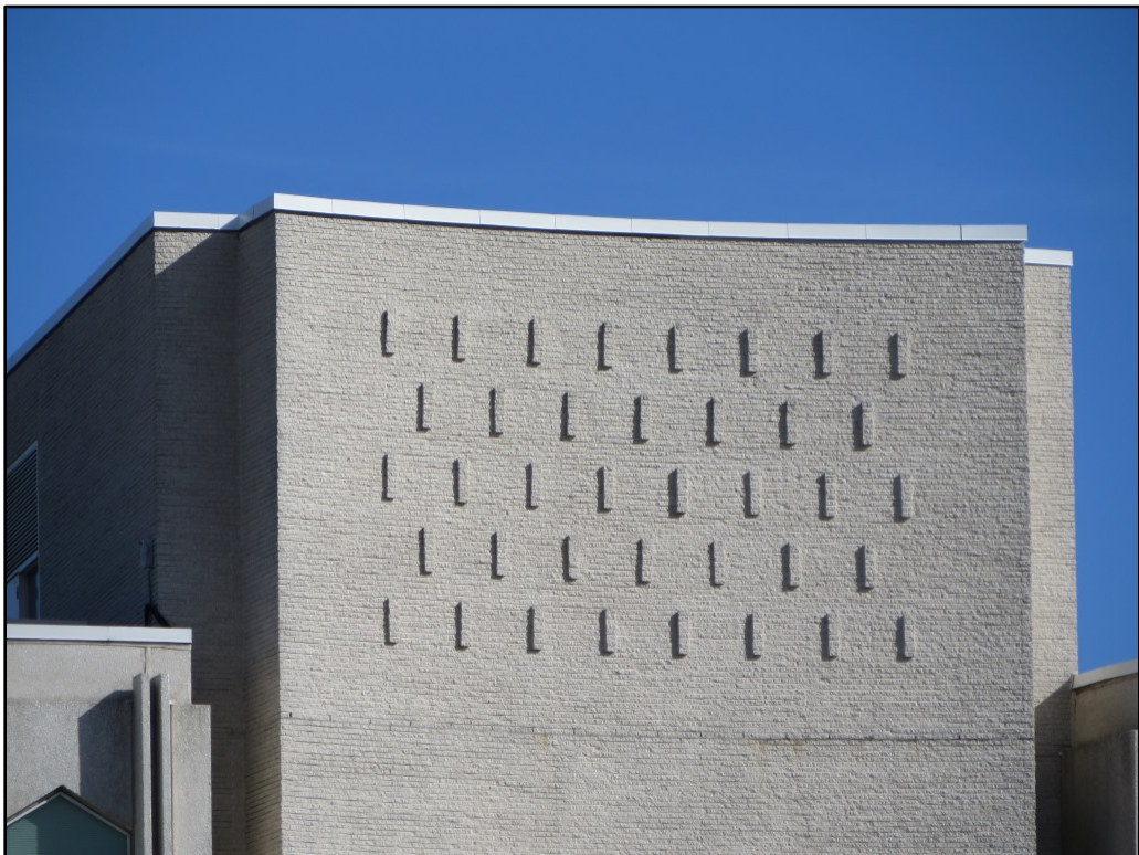
Photograph 20. Detail view of typical brickwork on the five four-story stairwell/elevator tower sections of the Office and Conference Center, view to east.
