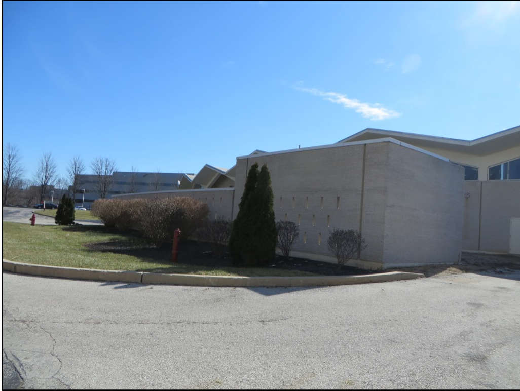
Photograph 31. Enclosed original utility area on the northwest side of the Graphic Arts Building, with ornamental pierced brick walls; view to south.
