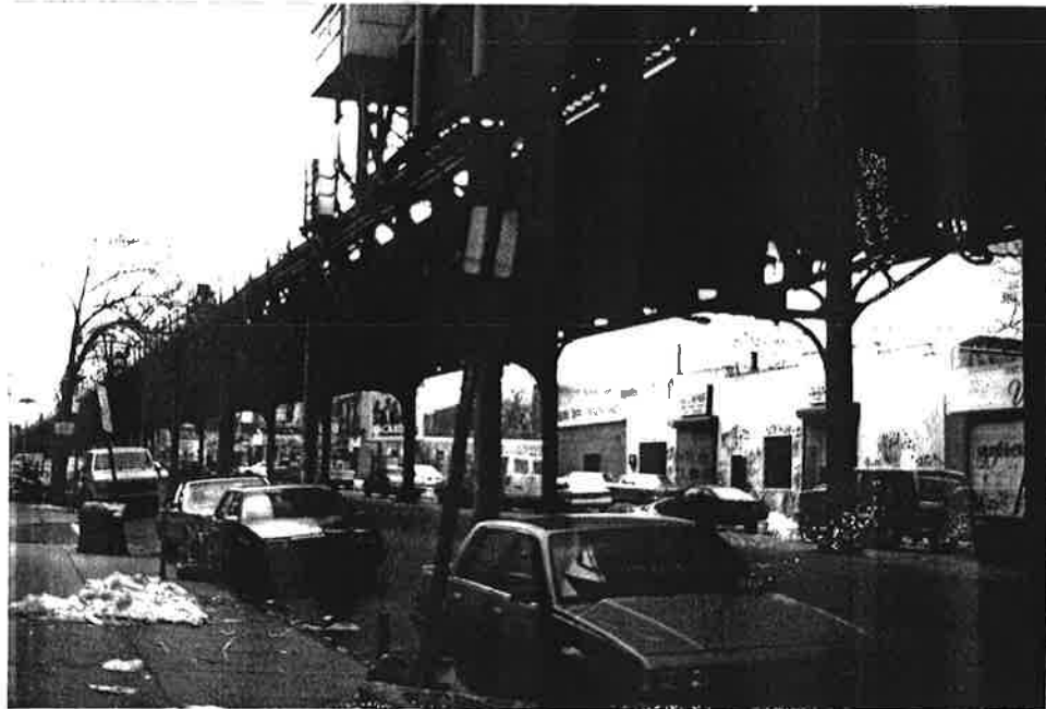
View of Elevated viaduct beneath 63rd Street Station. Note bracketed steel pillars and longitudinal lattice girders.
