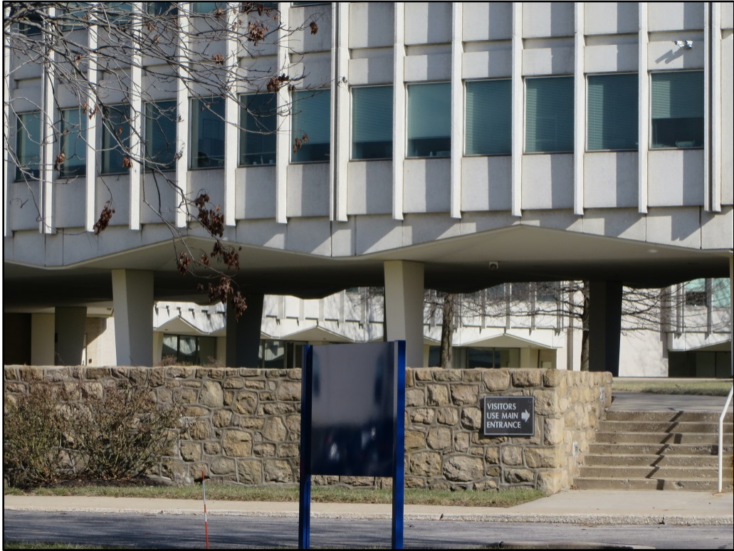
Photograph 11. Original stone retaining wall, concrete steps, and sidewalks along the west side of the Office and Conference Center, view to east.
