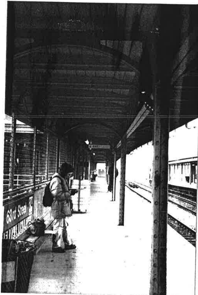
View of eastbound platform at 63rd Street Station. Note bracketed metal posts which support platform shelter.
