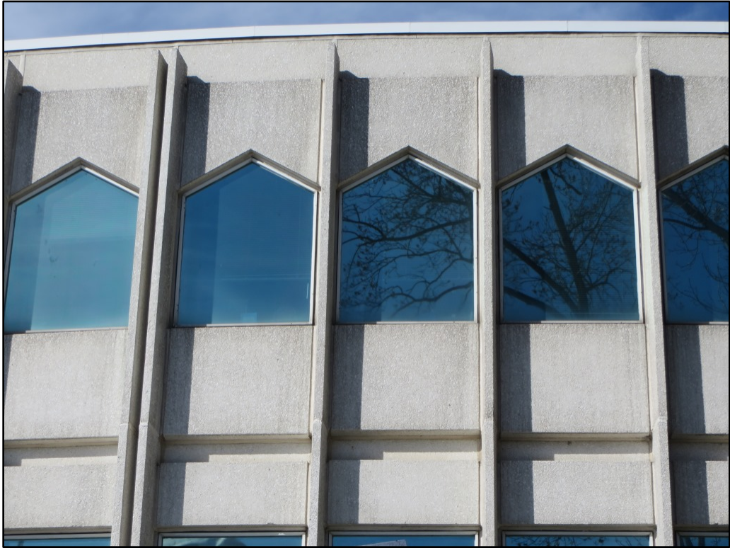
Photograph 19. Detail view of second-story windows in the south exterior elevation of the Office and Conference Center, looking northeast.
