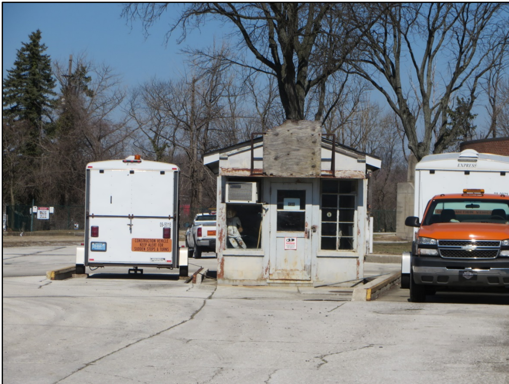
Photograph 6. View looking northeast toward the south elevation of the circa-1955 scale house.
